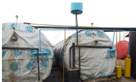
Fig.1. Biogas plant: 1 container for pre-treatment of biomass to be loaded; 2-tank for heating and loading; 3-bioreactor; 4-filtration of biogas; 5 - gasholder; 6-heating boiler
