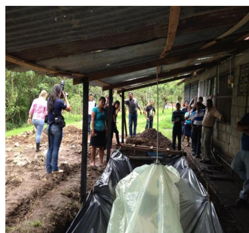
Photo 3. Biodigester finished. Photography: C. Saborío
