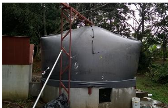
Photo 4. Flexible structure biodigester fully operational. (Taken from Carlos Saborio's investigation)
