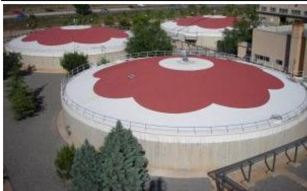
Photo 3. Fixed dome or Chinese biodigester fully operational. (Taken from AEBIG.com) .
