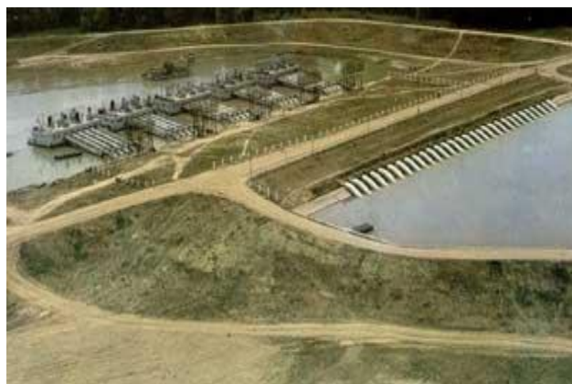
Photo 1. Floating pump station - Irrigation system Gălățui-Călărași
