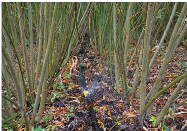
Photo 1. Irrigation pipe, with outlet point, laid in an actively growing SRC willow planta
