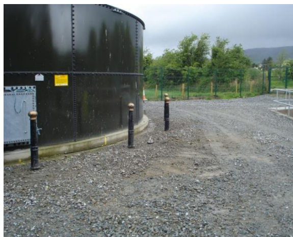
Photo. 2. Holding tank at Bridgend WWTWs, Co. Donegal, Republic of Ireland
