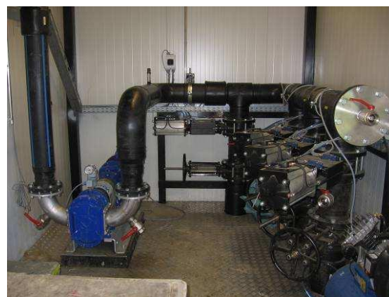
Fig. 3. Pumping systems (AGRINZ 2008)
